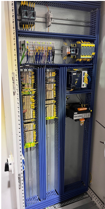
Figure 2A: Nice electrical cabinet
