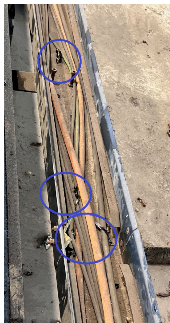
Figure 3A: Metal chips inside cable tray
